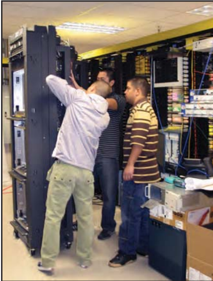
CENIC NOC Engineers in the process of removing end-of-life optical equipment as part of the CalREN backbone update.
